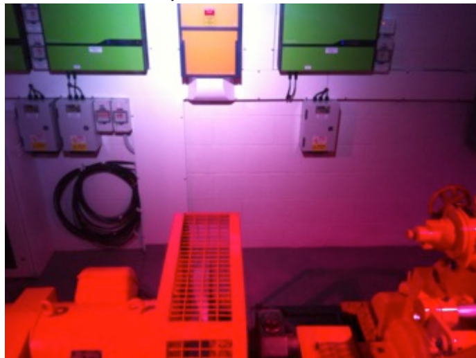
Steveanson Falls – Hydro-Electric Turbine
